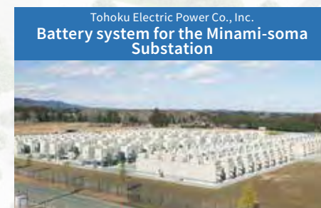
Tohoku Electric Power Co., Inc. Battery system for the Minami-soma Substation This battery has been adopted for measures to balance the demand and supply due to diffusion of recyclable energy.
