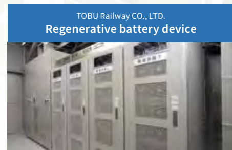
TOBU Railway CO., LTD. Regenerative battery device This battery has been adopted for regenerative battery devices to effectively use the regenerative electricity generated by deceleration of a railcar.
