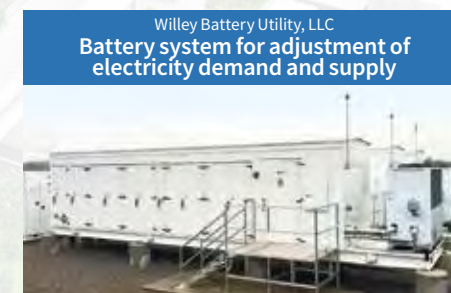
Wiley Battery Utility, LLC Battery system for adjustment of electricity demand and supply This battery has been adopted for large battery systems for adjustment of electricity demand and supply in the United States.
